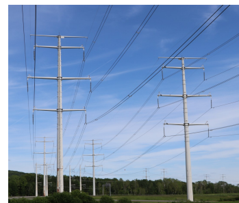
Figure 1.1 345,000 volt transmission lines.
